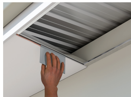
Step 3. Butter the edge of the 1st sheet with a thin layer of the epoxy. Take note to mix only a small amount of Epoxy to avoid wastage due to premature hardening.
