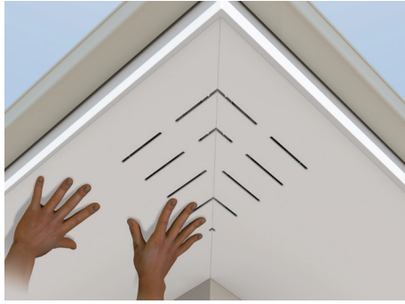
Step 5. Repeat the same procedure as before for the other side of the mitre cut. DO NOT FIX immediately the 2nd mitered sheet.
