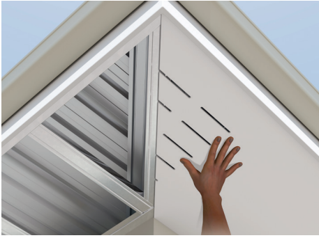
Step 4. Fit the mitered sheet and once certain of the fit, fix according to design table and sheet edge fastening recommendations.
